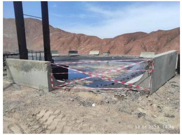
Photo 77. Production base of AC plant. Completion of full fencing of bitumen storage area is ensured.
