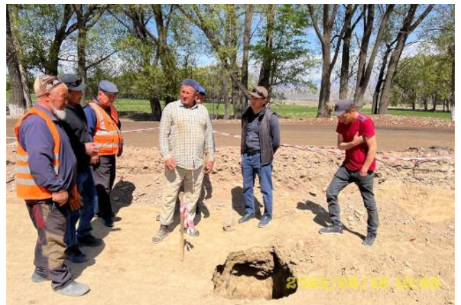
Photo 128. Lot 2. Km. 62+500. v. Tendik. Inspection by Consultant and Imam of found burial site.
