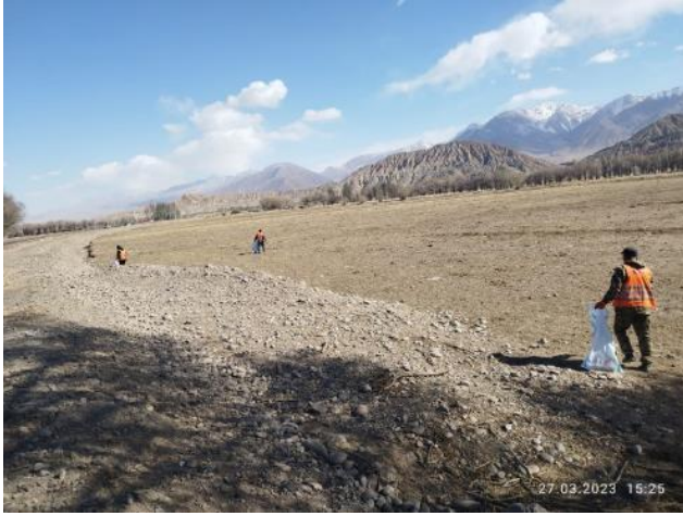
Photo 82. Lot 2. March. Sanitary cleaning of the area along the project road at km 63+480
