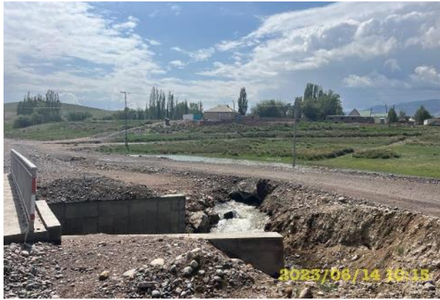
Photo 110. Bypass road of the bridge at km 86+261. r. Sazdyn-Suusu,. Construction of the bridge is completed; the bridge bypass is open. The bypass road is subject to reclamation.
