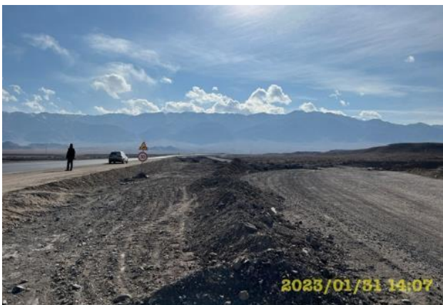
Photo 66. Lot 1. Bypass road on the section km. 22+000-23+000. Subject to reclamation.
