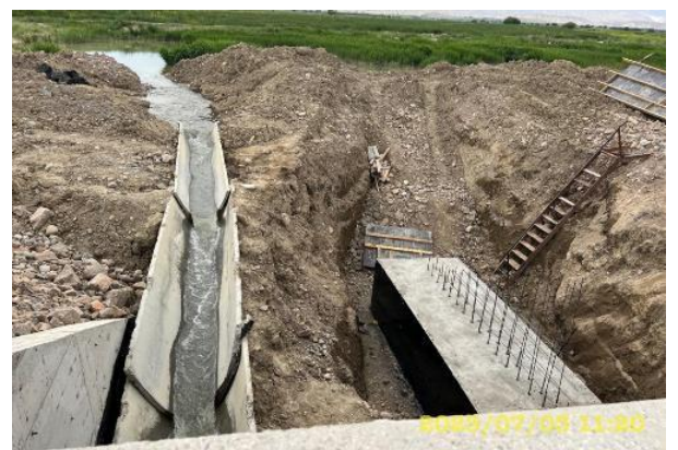
Photo 109. Mukandyn-Suusu river bridge, km. 68+040 It is necessary to provide water diversion measures to prevent soil from entering the river during construction works.
