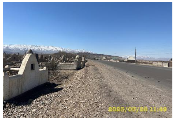
Photo 87. Lot 2. March Cemetery km 68 road LHS: after clearing sections of grave fences from backfill soil.
