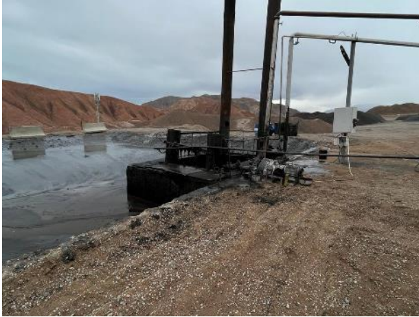
Photo 76. Production base of AC plant. Fencing around the bitumen storage area to be completed
