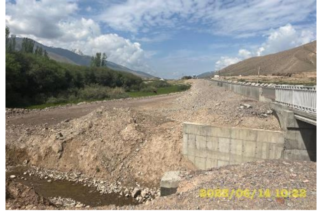
Photo 111. Bypass road of the bridge at km 88+795. r. Zhar-Korundu. Construction of the bridge is completed; the bridge bypass is open. The bypass road is subject to reclamation.
