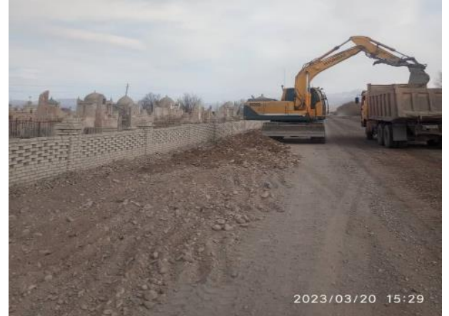
Photo 85. Lot 2. March. Cemetery km 68 road RHS: area along cemetery fence cleared of backfilled soil
