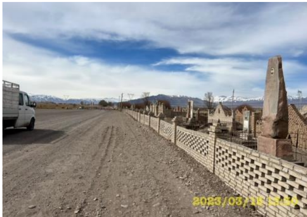
Photo 84. Lot 2. March. Cemetery km 68 RHS, foundation of cemetery fence along road is backfilled with soil as a result of roadside construction.
